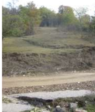
Figure 14: Landslide and damaged road
